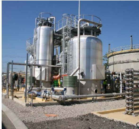
Fig. 1.3 Sludge thermal hydrolysis plant
